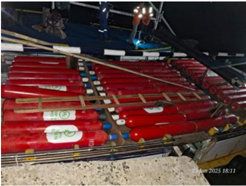
Figure 3. Hydrogen Distribution to Gili Ketapang Diesel Power Plant
