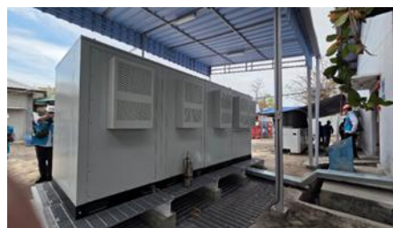
Figure 5. BESS at the Gili Ketapang PLTD
